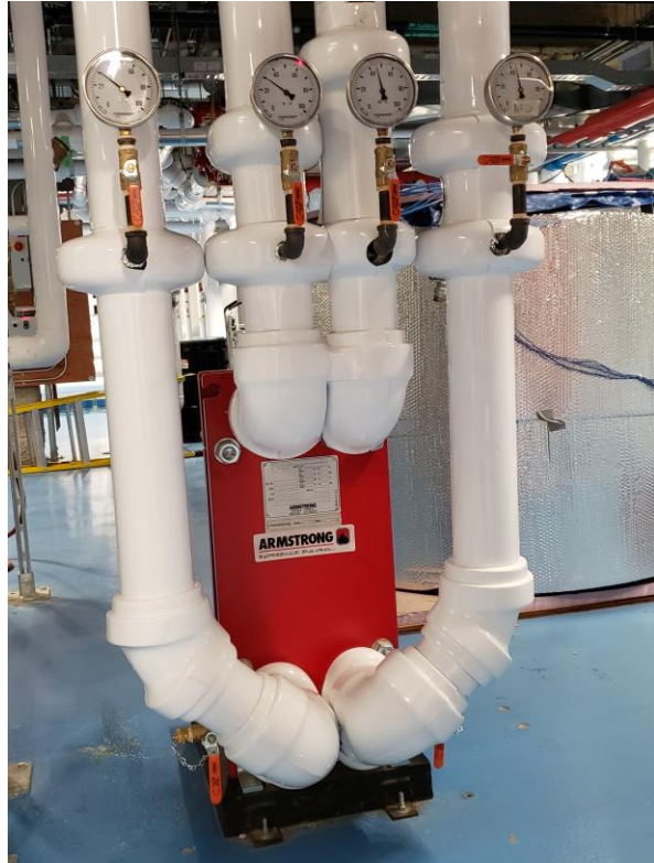
Typical Energy Transfer Station
